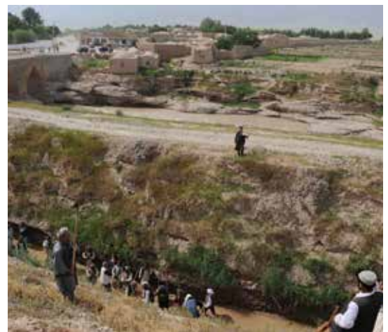
Mazar-e-Sharif, Northern Afghanistan. Dredging a mirhab irrigation canal on Balkh River near Mazar-e-Sharif in Northern Afghanistan. Such systems, primitive they may seem, are still instrumental in feeding the country. Balkh River and Kholm River ceased to flow into Amu Darya centuries ago, extensive irrigation may have seriously contributed. The DelPHE project strives to turn the mirhab networking into a broader environmental stewardship system, not just water management as it always was.
